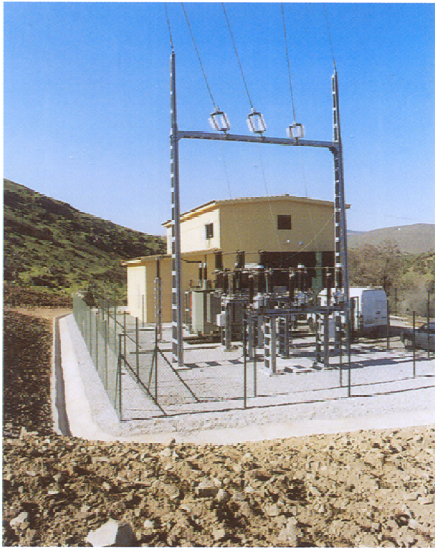
Powerhouse and substation
