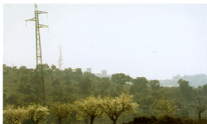
Line interconnecting the grid
